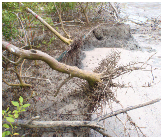
Fig. 4. Widespread uprooting and collapsing of trees in T2 (without geotubes)
