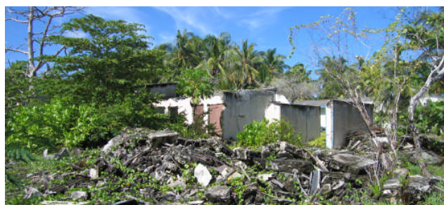
Fig. 1. House on Madifushi damaged by tsunami
